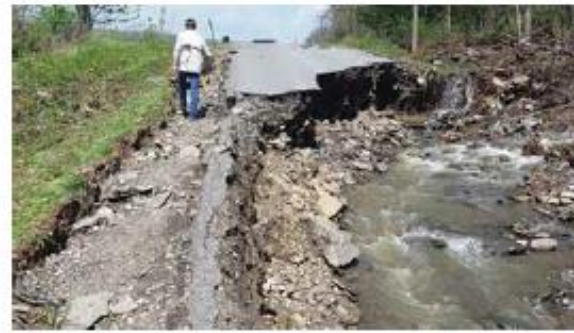
East Valley Road, north of Branchport, NY. Floodwaters were beyond the capacity of existing ditches and culverts. Many area roads were damaged from the velocity and volume of the floodwater. Photo: Courtesy of Dave Enty (NWS Binghamton).
