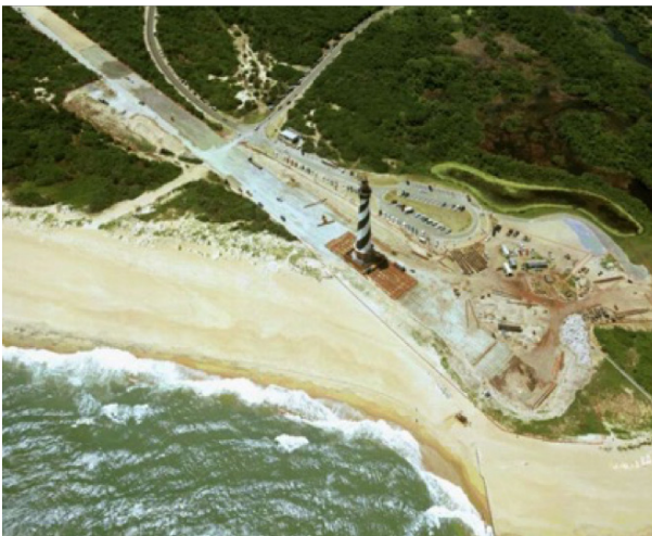
The National Park Service relocating the Cape Hatteras Lighthouse, National Seashore North Carolina. Photo from: NPS
